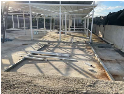
Concrete land with roof (Application No. A/YL-KTS/906, photo taken on 29/05/2024)
